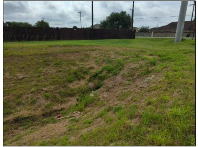
Photo 6. Drainage ditch with structure inlet north of FM 2480 (Old Port Rd), viewing southeast
