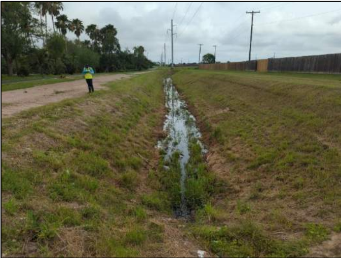
Photo 11. Drainage ditch with standing water north of existing structures, viewing north
