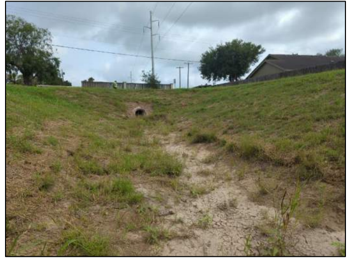
Photo 2. Bottom of drainage ditch with structure outlet south of FM 2480 (Old Port Rd), viewing north
