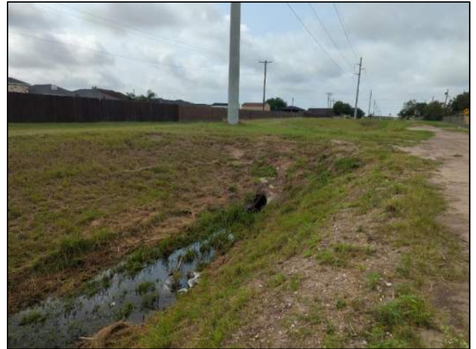
Photo 12. Existing structure inlet with standing water in drainage ditch, viewing southeast
