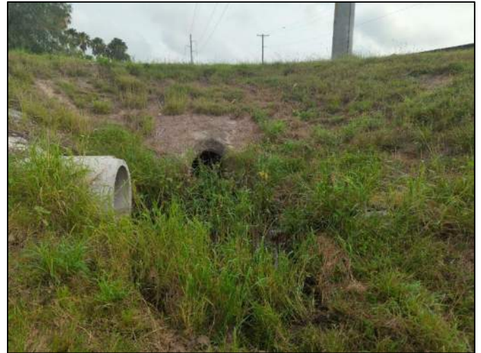
Photo 8. Drainage ditch with standing water at existing structure outlets, viewing north
