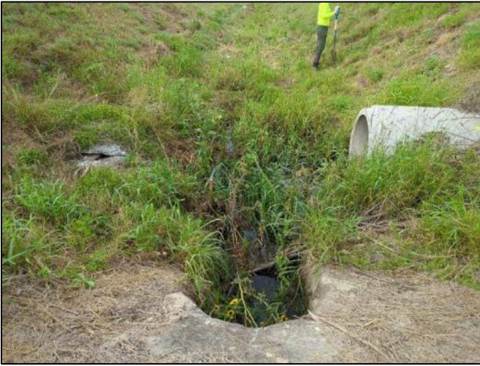
Photo 9. Drainage ditch with standing water at existing structure outlets, viewing south
