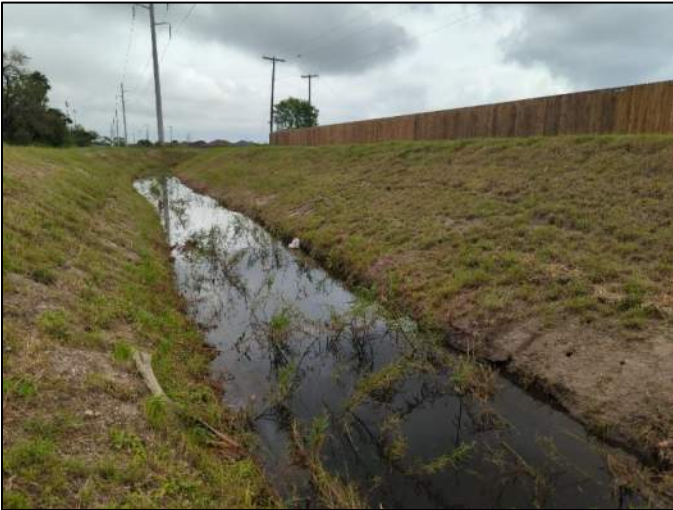
Photo 13. Drainage ditch slopes with standing water in bottom near proposed new structure outlet, viewing northeast
