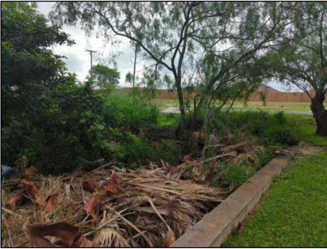
Photo 17. Plant debris at proposed new structure inlet location with retaining wall along adjacent residential property, viewing east
